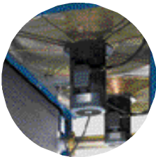
Plant cooling fan. The cool air passing through the unit picks up all radiant heat
